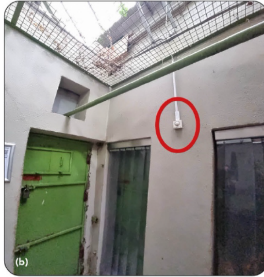
Figure 13.03: (a) The sloth habitat, note the glass roof component of the enclosure (challenging to maintain temperatures) and the location of one of the temperature and humidity dataloggers (red circle); (b) the ambient heating system is controlled by the thermostat which is located in the keeper area, outside of the actual habitat but in a shared airspace.
